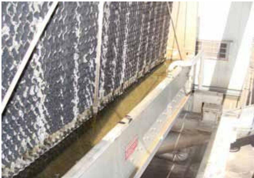
PHOTO 3. Side/top view of cooling tower basin showing water in basin.
