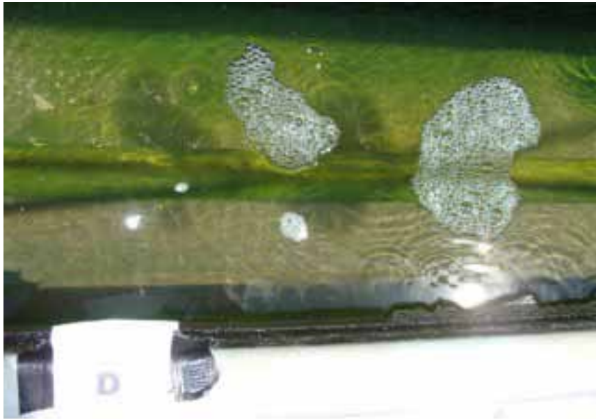
PHOTO 4. Day 1, site D. Algae in basin and coating PVC pipe prior to Solution 3000 application. Direct measurement of the algae deposit was not possible since it washes away when disturbed, due to the flow of the water.
