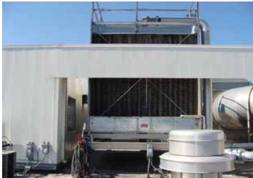
PHOTO 1. Cooling tower general view.
