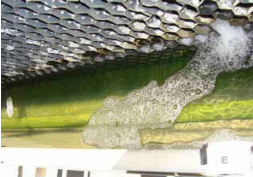
PHOTO 14. Day 1, Site E, prior to Solution 3000 application. This site was in the same basin as site D, in the middle of the basin approximately 7 feet away.
