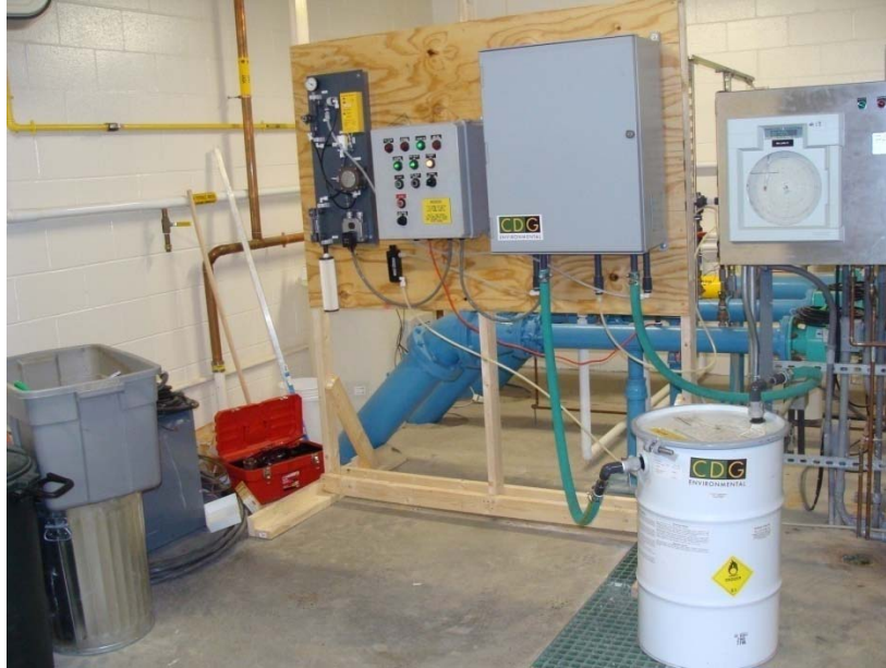
Figure 1 CDG Gas:Solid chlorine dioxide generator at the Canton pump station. The Saf-T-Chlor drum (white) is shown in lower right.
